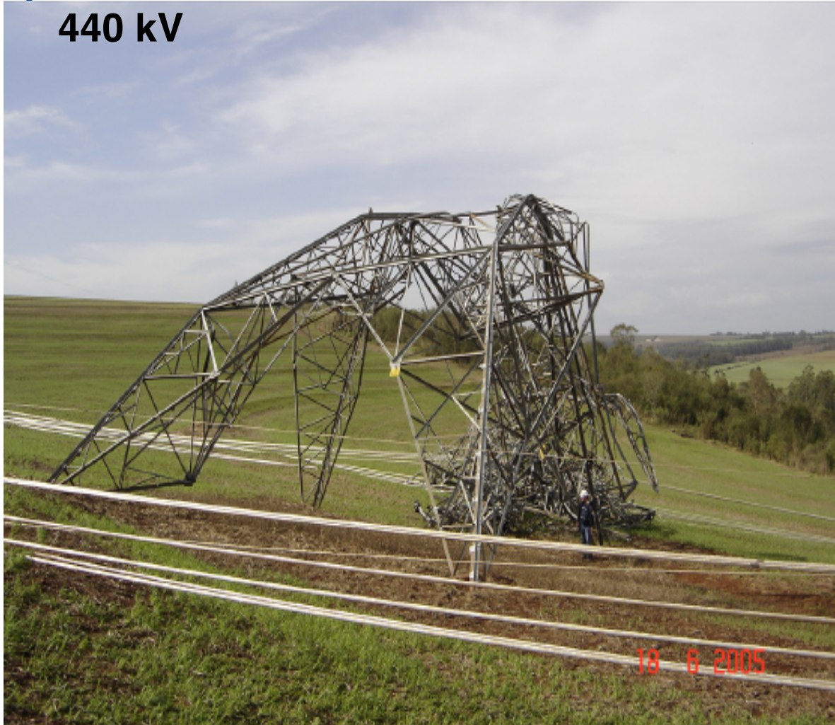
765kV Itaipu Transmission System - Photo from FURNAS
